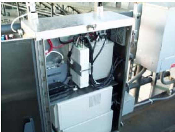
One of the three panel-mounted data acquisition stations (See block diagram on next page)
